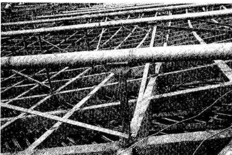
Fig. 4.12 Detail of CHS rafters supported on angle struts fixed to lattice beam
