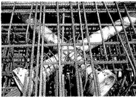
Fig 2.4 (a) Anchorage blocks of cable net above the surface of the ring beam
