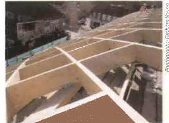
The curved roof of Hounslow East tube station is formed of an elegant diagrid structure of Kerto LVL beams connected together in a lamella sequence. The Kerto beams were bolted together with a 'Cowley' connector.
