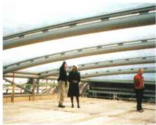
An ETFE atrium roof is set between curved steel tubes supported by steel 'tree' columns. Adastral House, London.
