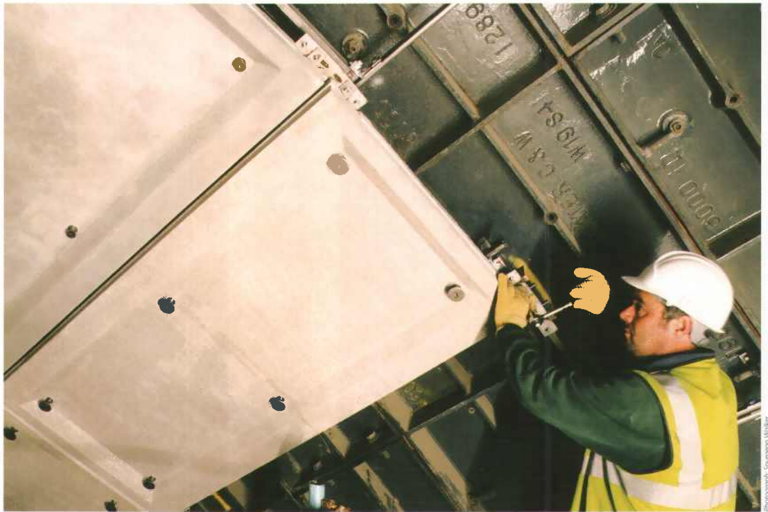
The steel-lined tunnel which serves the Heathrow Express high-speed rail link is lined with coffered GRC panels.
