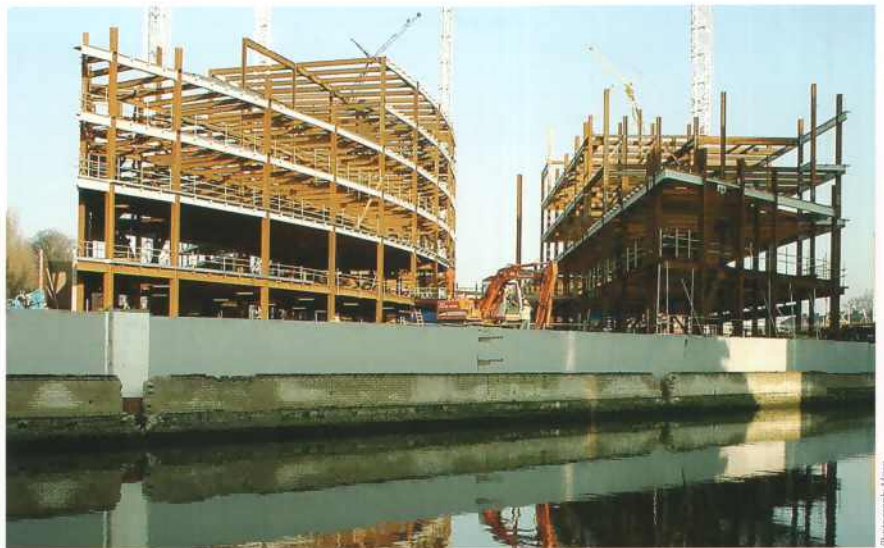
GSK House during construction. The white intumescent-coated edge beams are clearly visible.
