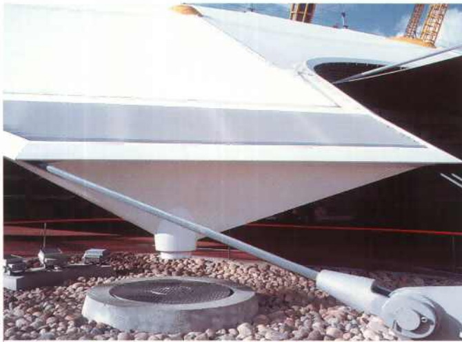
HOPPERS COLLECT RAINWATER VIA A PERIMETER GUTTER AND DISCHARGES INTO THE UNDERGROUND SYSTEM
