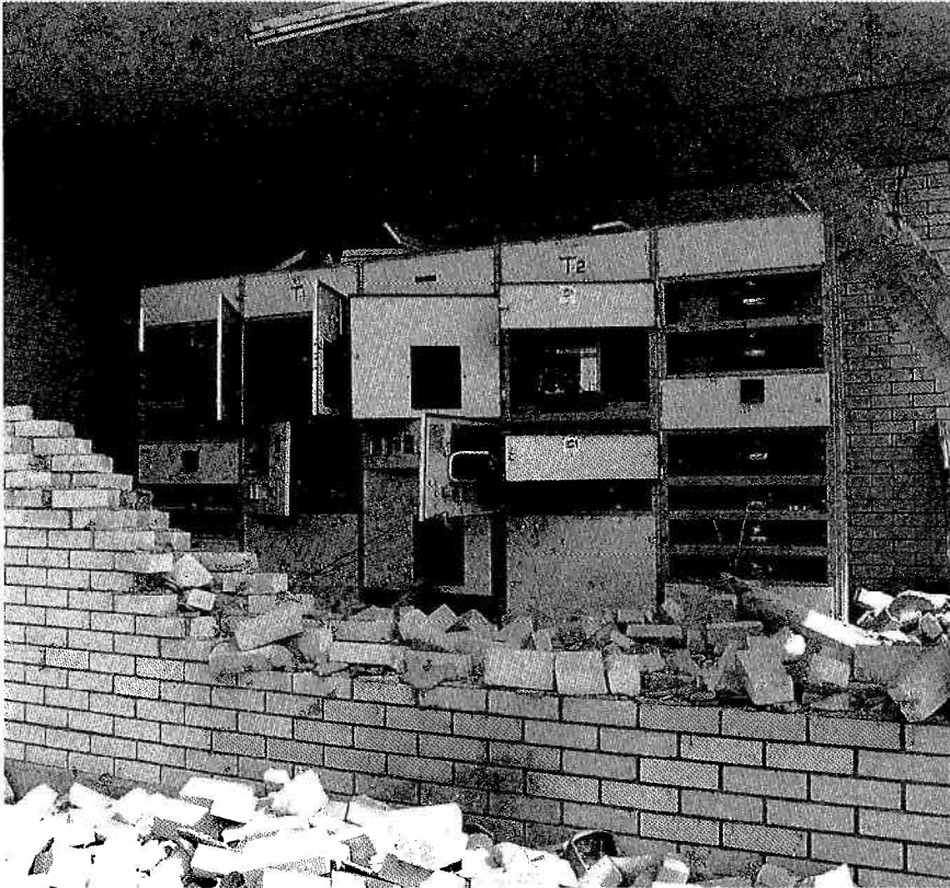
Fig 7.21 Destruction of walls and structure of substation, and of switchgear
