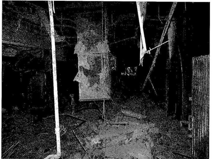
Fig 7.4 Fire damage inside Souk Al Kabir
