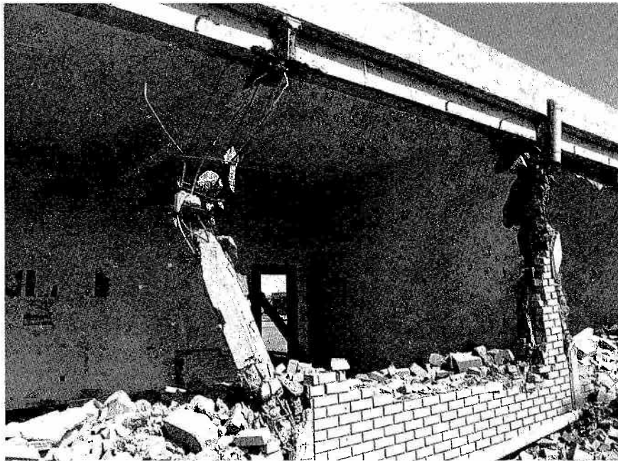
Fig 7.9 Destruction of walls and columns by tracked vehicle - MOD complex
