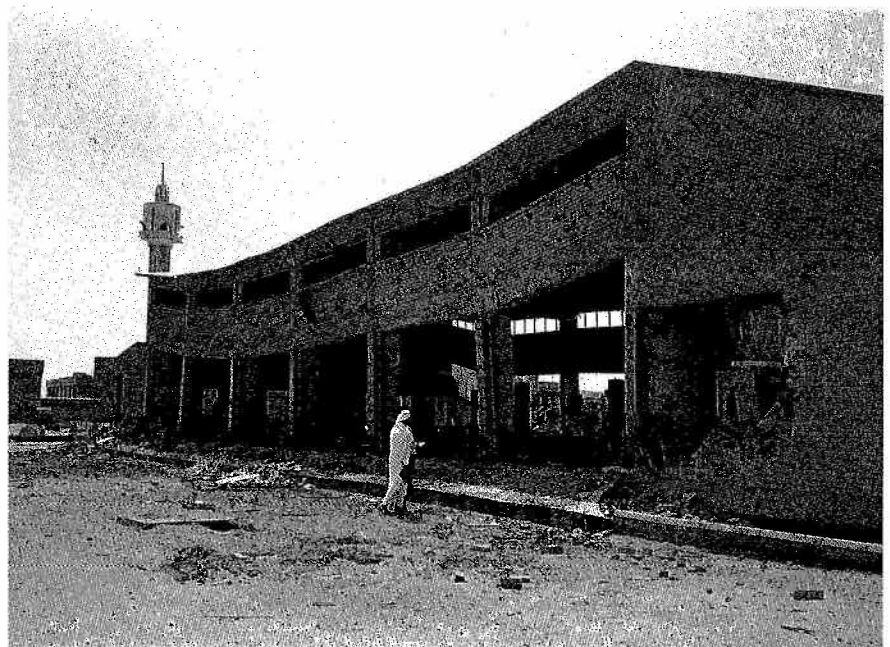
Fig 7.11 Explosive damage at base of columns in maintenance building of MOD complex
