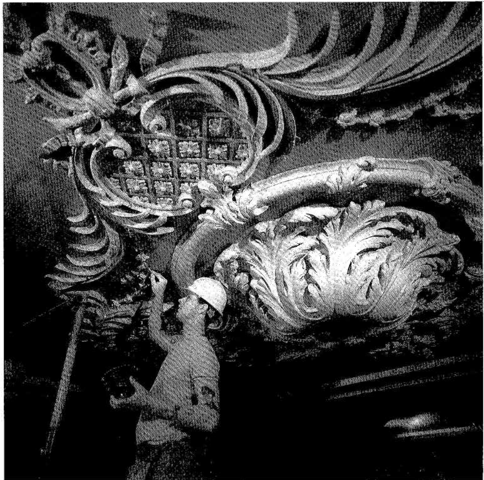
Fig 3.6 Fallen plasterwork of ceiling rose
